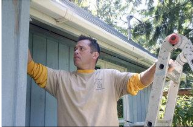
Navy Chief Petty Officer Rusty Vonqueruer, one of 19 volunteers from Naval Air Station Whidbey Island, helps paint a Scatchet Head cottage recently donated to Saratoga Community Housing for its Community Land Trust program.
